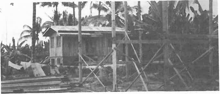
Beginning construction of the final building. It is being used now but not complete. Background--classroom, dormitory and library space.
